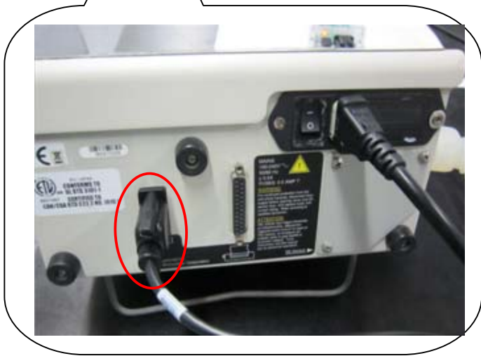
Cable connections at the calibration device (VT Plus ) end
